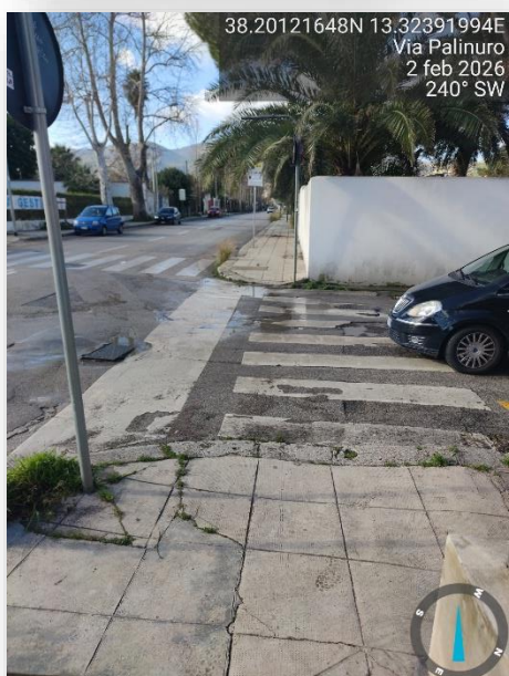
RAMPA INADEGUATA/ DISLIVELLO
