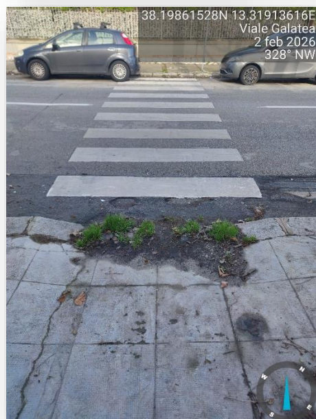
RAMPA INADEGUATA/ DISLIVELLO
