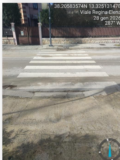
RAMPA INADEGUATA/ OSTACOLI
